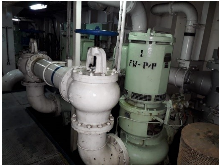
Gambar 2. Pompa Air Tawar
