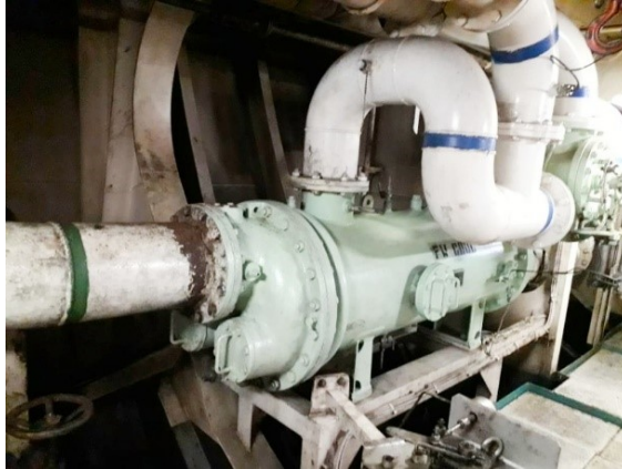
Gambar 3. Fresh Water Cooler
